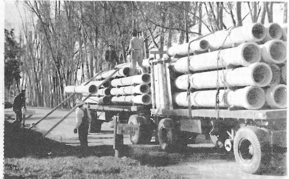
TRUCK AND TRAILER UNLOADING 10 AND 14 INCH PIPE ON TAVERN ROAD. MAN WITH ROPE ALLOWS 400 POUND PIPE TO ROLL DOWN ON STEEL RAILS.
