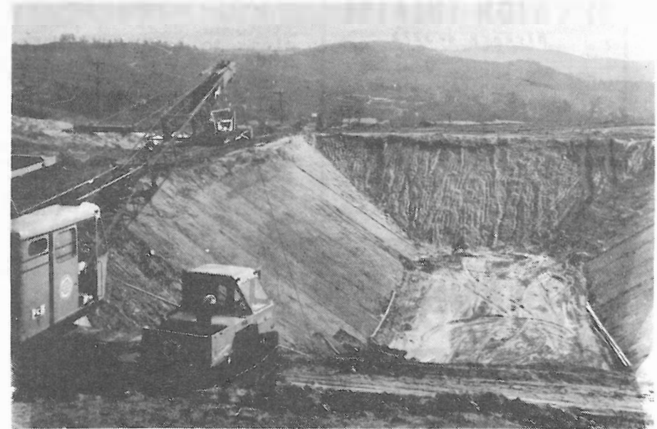
MAIN RESERVOIR ABOVE VILLAGE BEING SMOOTHED FOR POURING CONCRETE AND ROOF. NOTE 14 INCH PIPE AT FAR END. THIS WILL HOLD 2 MILLION GALLONS.
